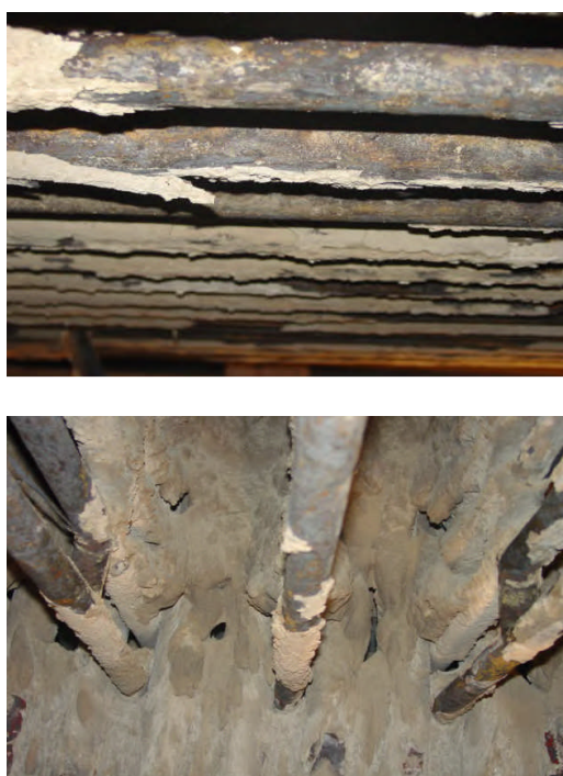
Figure 2.15: Fouling phenomena to tubing (up) and water walls (b) that lead to flaking and failure (Watson, 2008)
