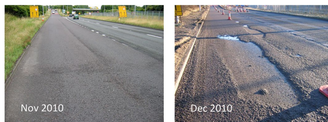
Fig. 1. Strategic road network in England: Rapid deterioration in road surface as a result of fretting, over the course of 1 month.
