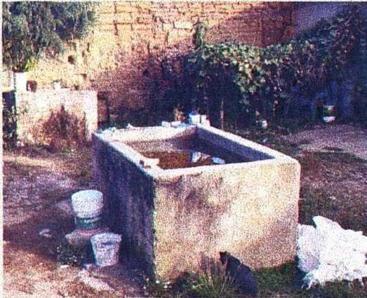
Figure 4.15. Domestic water reserve
