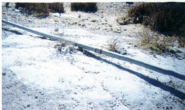
Figure 4.33. Open-air water supply pipe in Cholula 2
