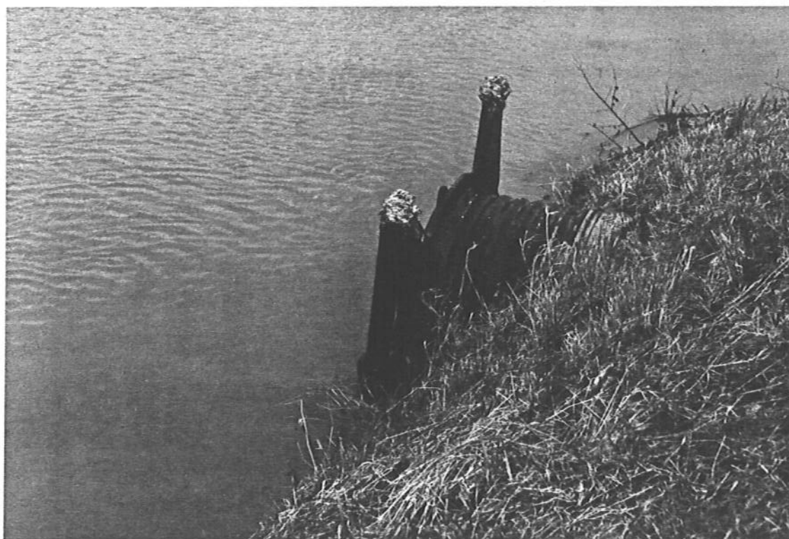
Plate 11: Outfall for Drain 23 near Mattersey - December 1992
