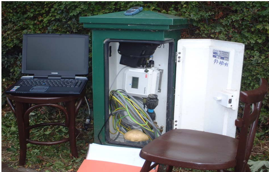
Figure 7.6: Site set-up for SAM 5year audit showing data collection system
