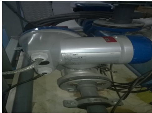
Figure 3.6: Sand/water Flow Meter connected to Pipeline from Sand Hopper
