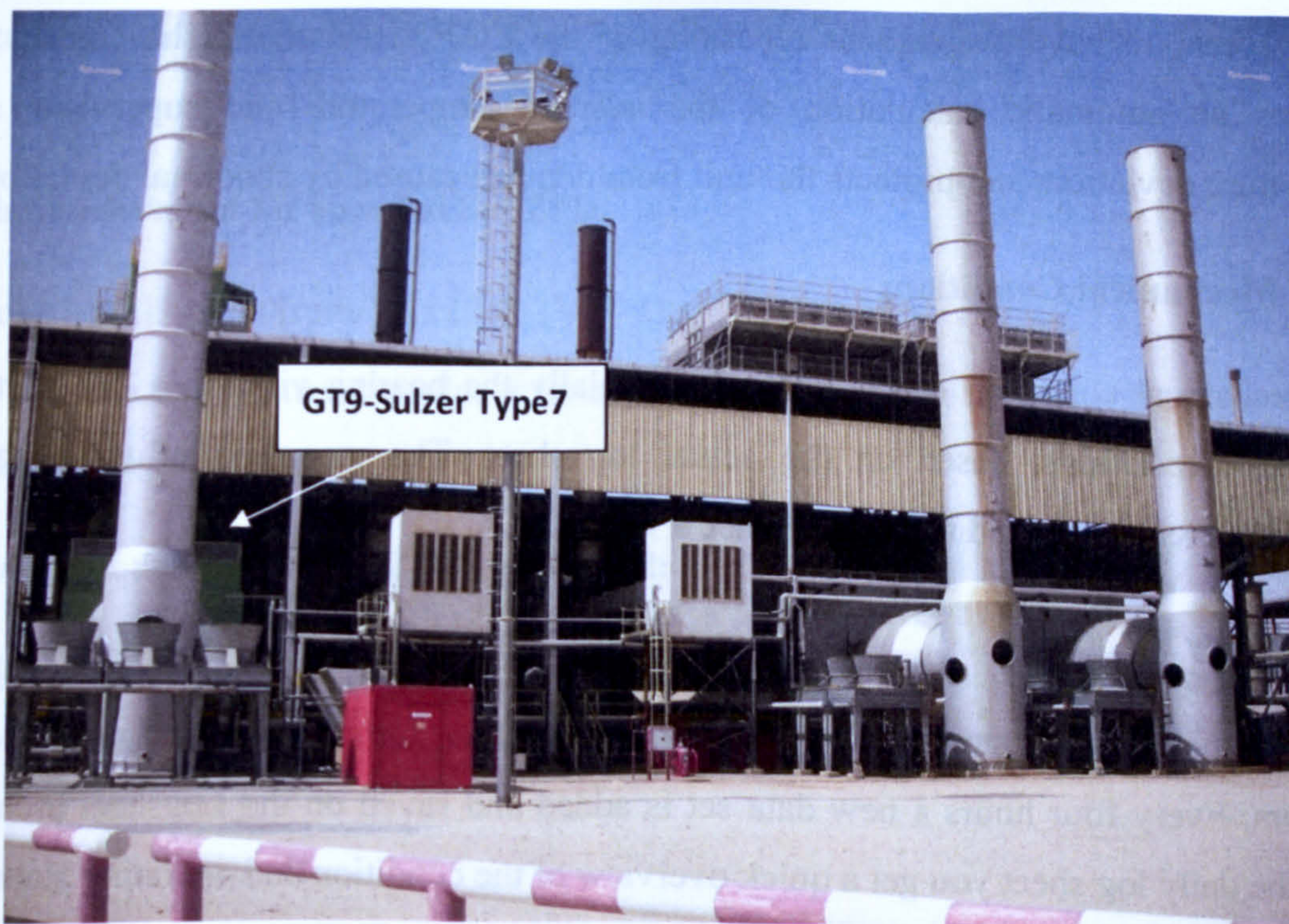
Figure 3-7: GT9 Power Plant (Courtesy of ENI Oil – Libyan branch, Abu-Attifel Field, 2008)
