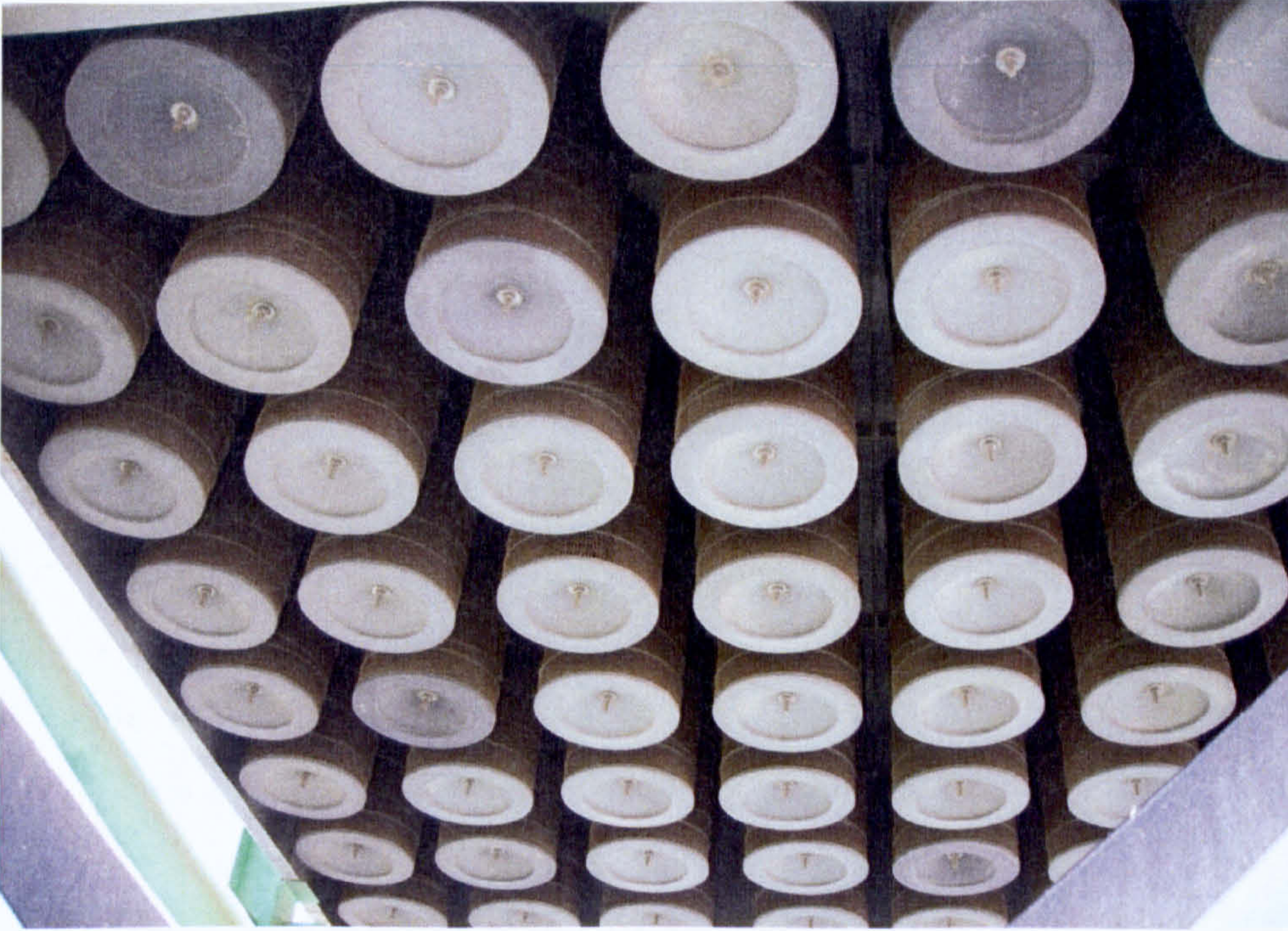
Figure 2-33: Self Cleaning Filters in a Desert Environment (Courtesy of ENI Oil – Libyan branch, Abu-Attifel Field, 2008)
