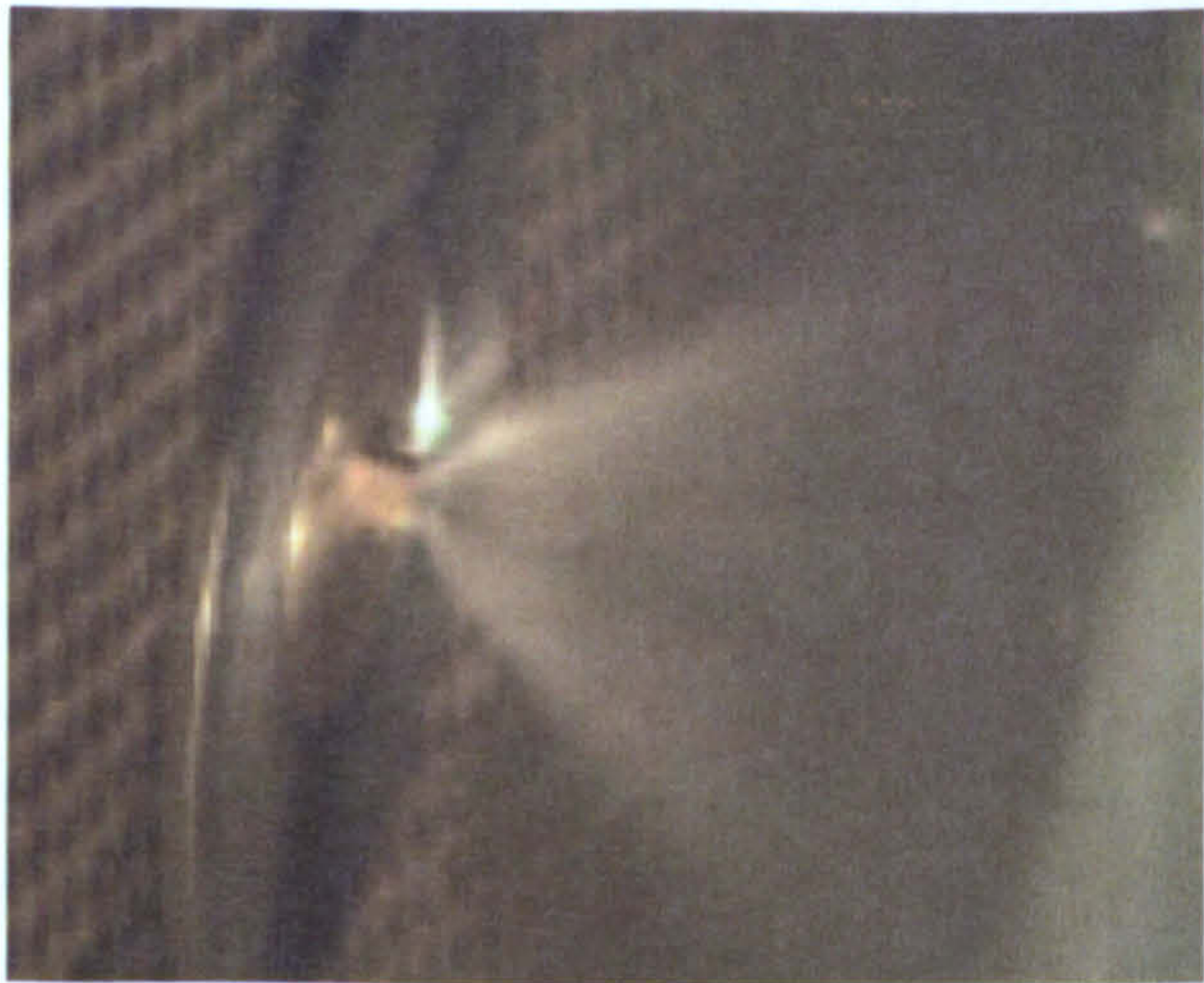
Figure 2-11: The water spray of the Mk3 on-line nozzle pictured at base load (Oosting, J. and Stalder, J. P., 2007)
