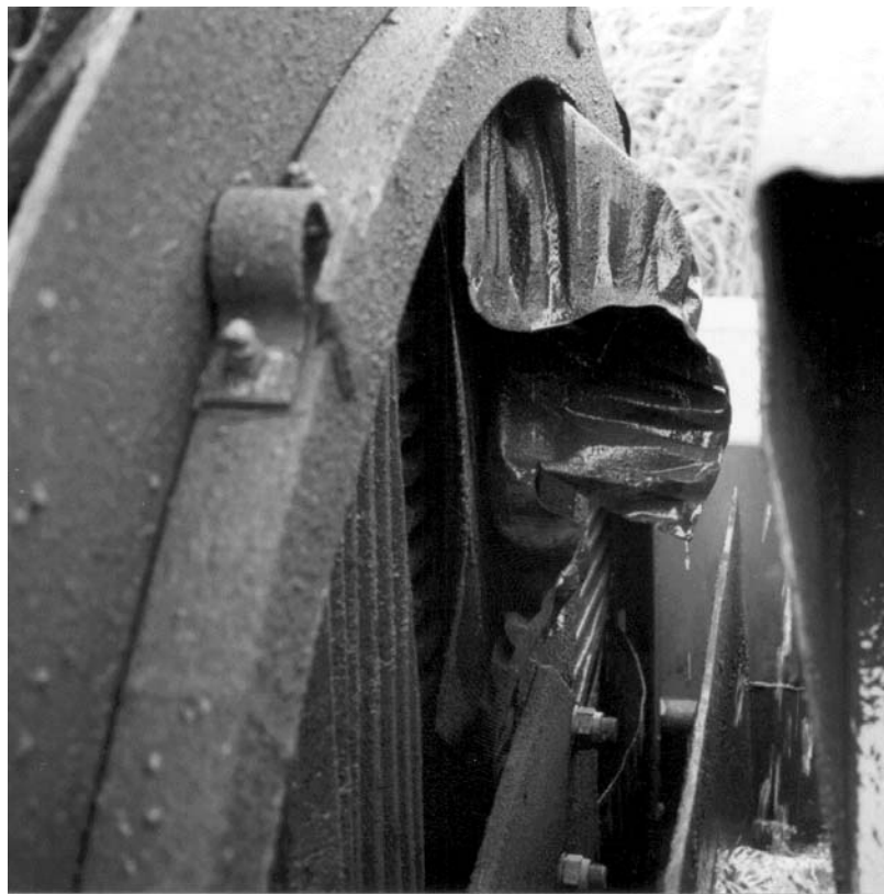
Figure 26 Crumbling of High density polypropylene media panels
