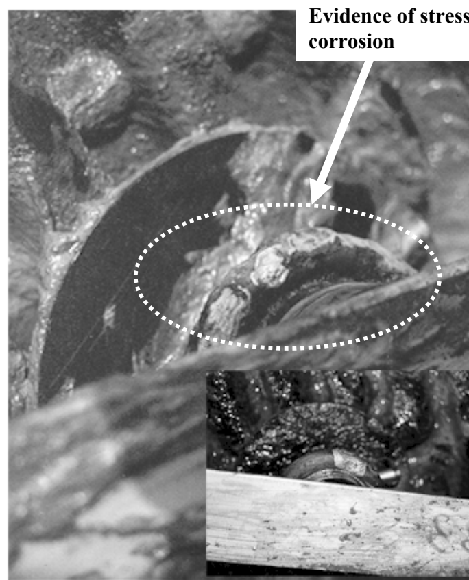
Figure 72 Stress corrosion of ‘U’ bolt
