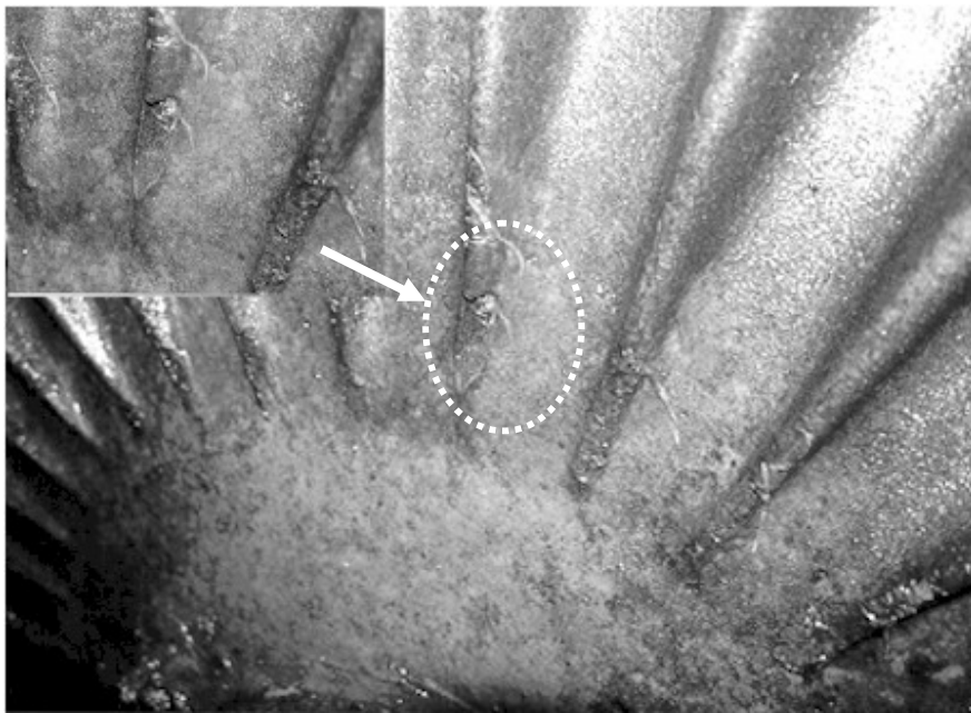
Figure 9 Early signs of GRP media disintegration
