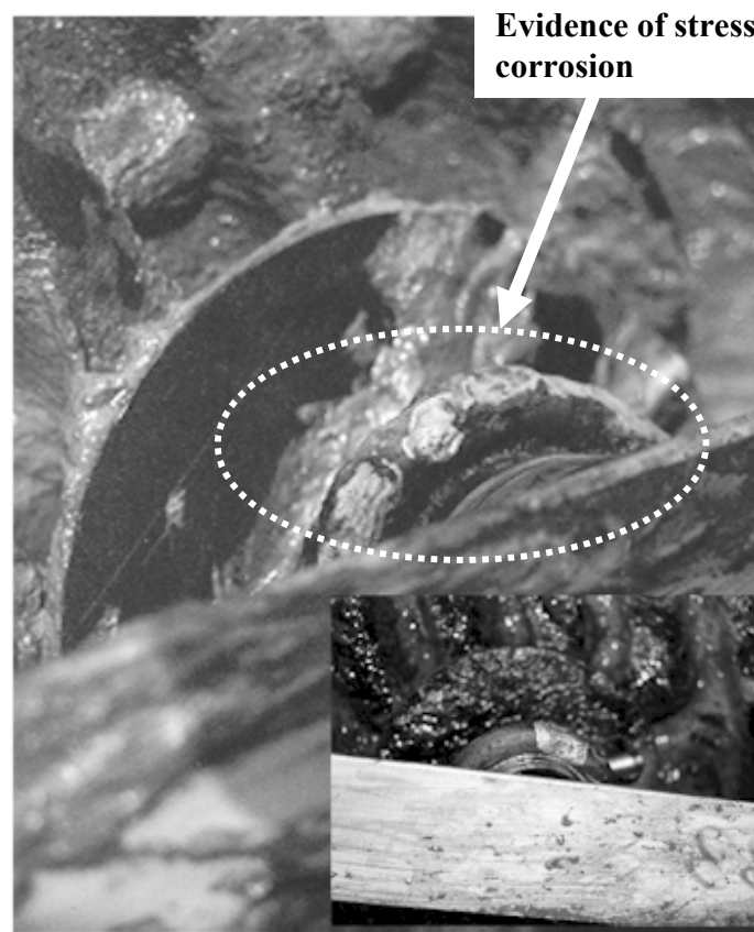
Figure 72 Stress corrosion of ‘U’ bolt
