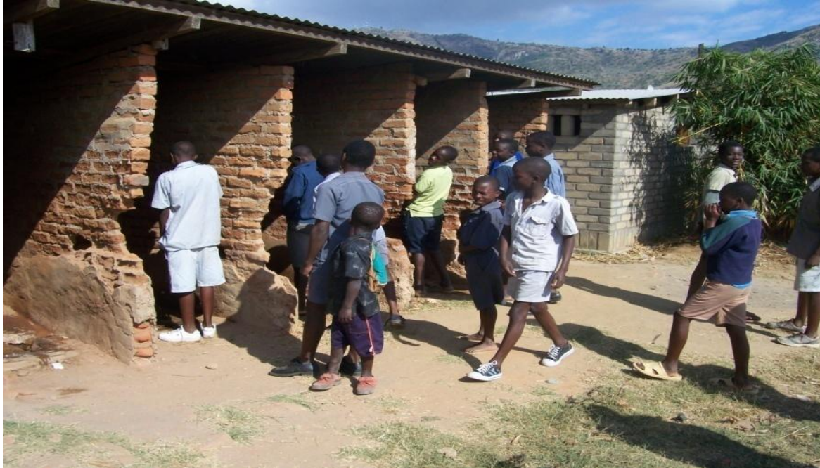
Figure 4. Damaged pit latrines still being used by pupils
