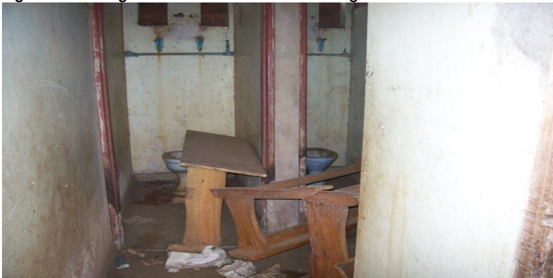
Figure 5. Damaged flush toilet used as a storage room
