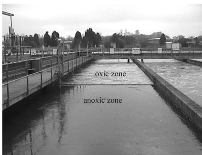
Figure 2: Activated sludge aeration lane at Finham
