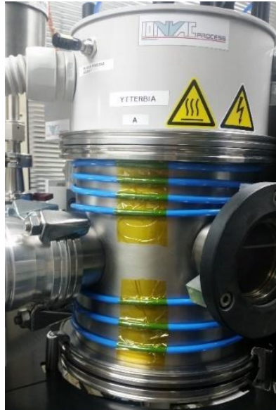
Figure 53: Water cooling pipes for temperature control.
