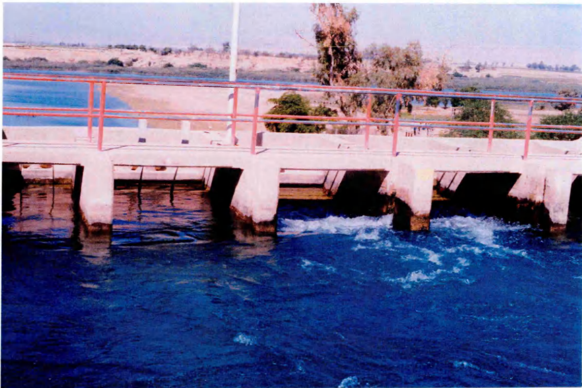
Figure 2-4. Pump station intake for the Sabilli area of the Dez scheme
