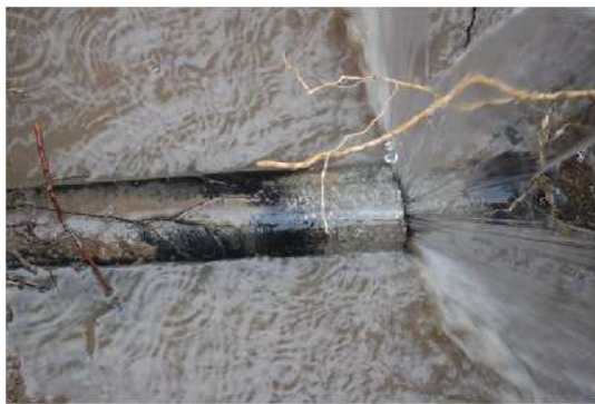
Circumferential break on an asbestos cement pipe.
