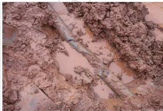
Longitudinal split on a polyvinyl chloride pipe.
