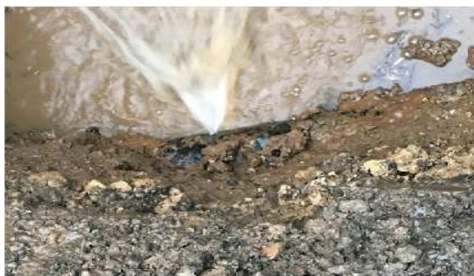
Corrosion pin hole on an iron pipe.
