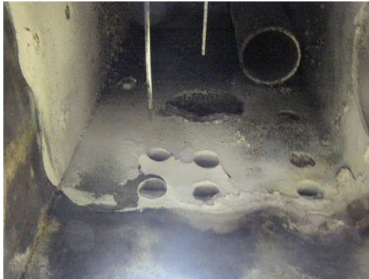
Figure E.2: Formation of fouling deposit (white colour) along internal walls of combustor during combustion of DDGS-MRFR (90:10). Tube located at top right of the photograph is the fuel “drop” tube as shown in Figure 3.5. Thin wires protruding into the freeboard are thermocouples as shown in Figure 3.7
