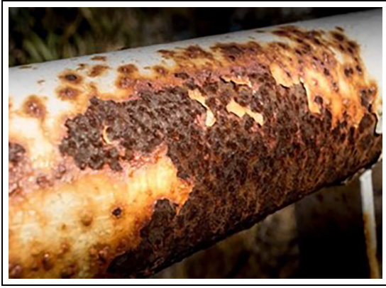
Figure 4. Corrosion in a pipeline and metal skin. 62
