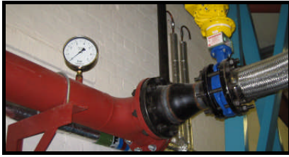
Figure 7.2: Pressure Gauge Upstream of UFR
