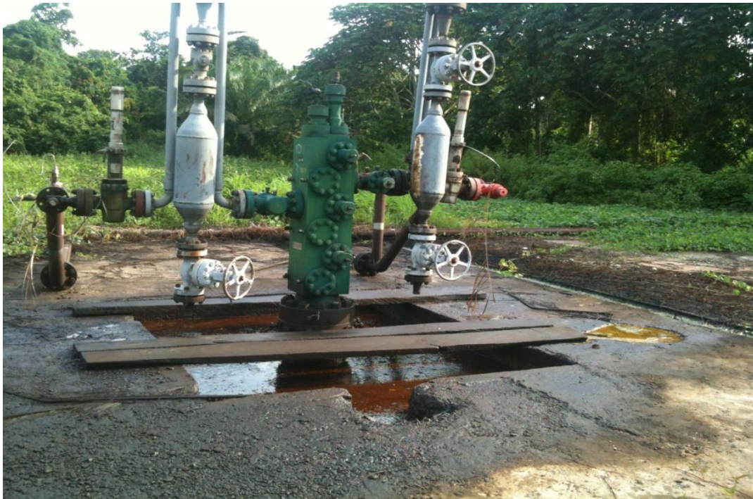
Figure 2-1. Well head in Biseni, Yenogoa, and site of oil spill
