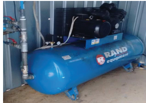
Figure 4. An air compressor system.
