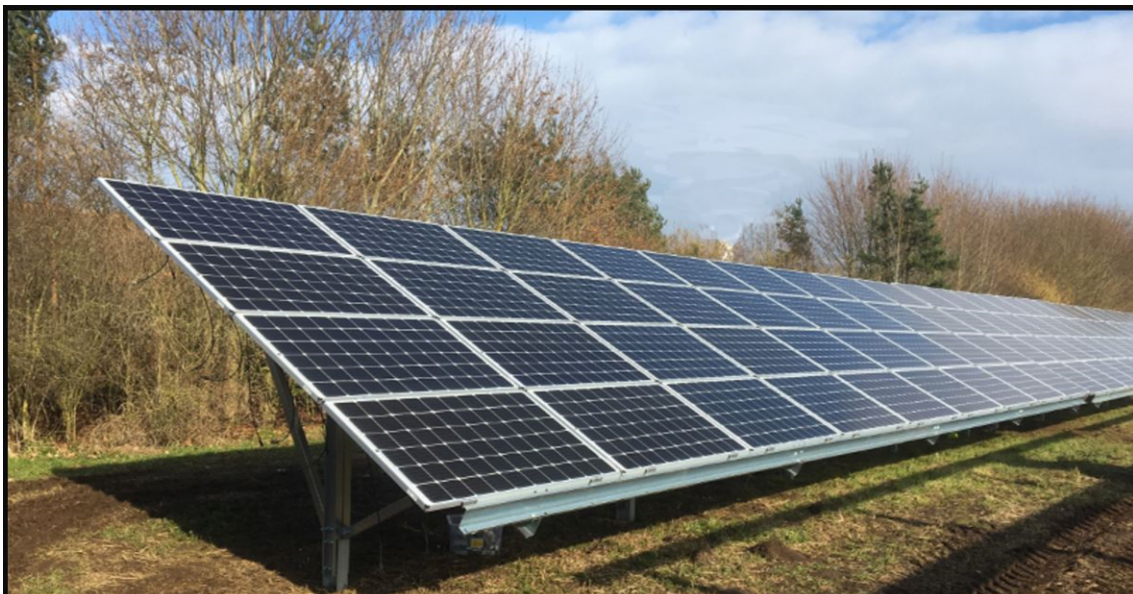
Figure 2-2 1MW solar farm installed in Cranfield Airport
