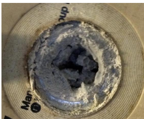
Figure 8-12 Calciner exhaust 90° angle bend blockage during attempted steam tests.
