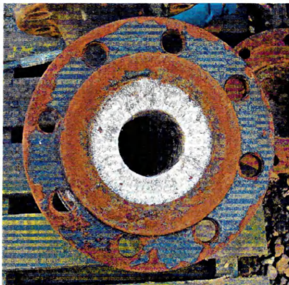
Figure A. Struvite deposition within a centrate pipe at Slough STW
