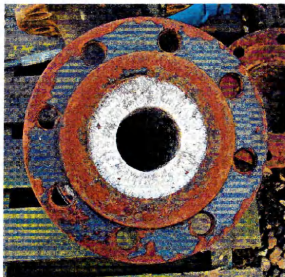
Figure 1.5 Struvite deposition within a centrate pipe at Slough STW
