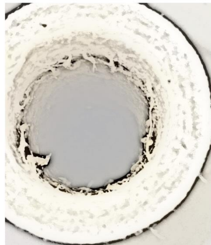
Filter after opening ball valve without an evacuation
