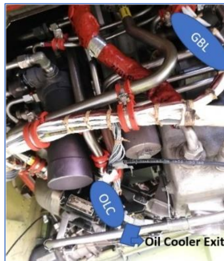
Figure 5-17 Location of GBL and OLC sensors with respect to oil cooler
