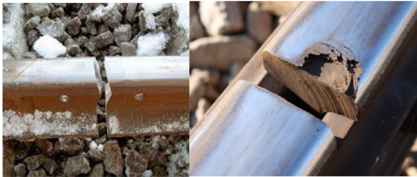
Fig. 3. Sample Rail track breaks.
