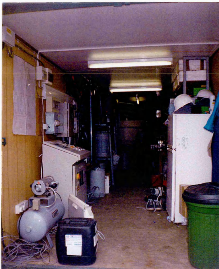
Plate 2. Pilot Plant Clarifier and Container
