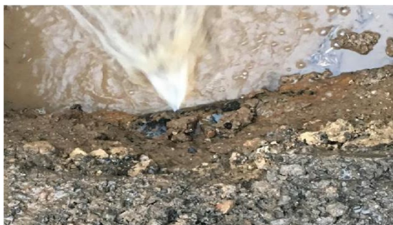
Corrosion pin hole on an iron pipe.
