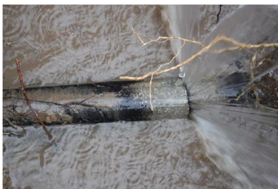
Circumferential break on an asbestos cement pipe.
