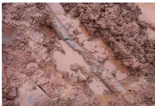
Longitudinal split on a polyvinyl chloride pipe.
