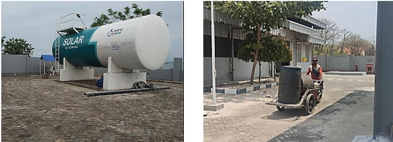
Figure 7. The Diesel Power Plant on Gili Ketapang.
