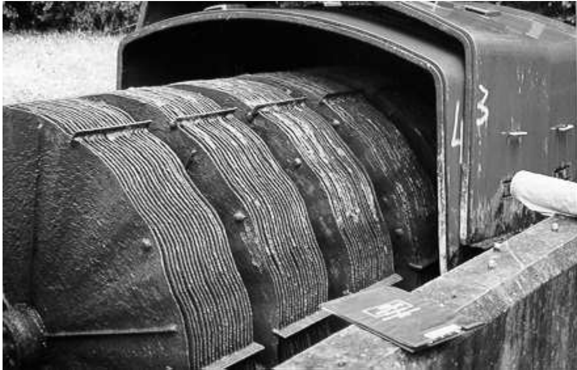
Figure 1 Rotating Biological Contactor
