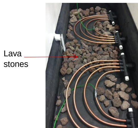
Figure 97: heat storing material o the basin area (Lava stone)
