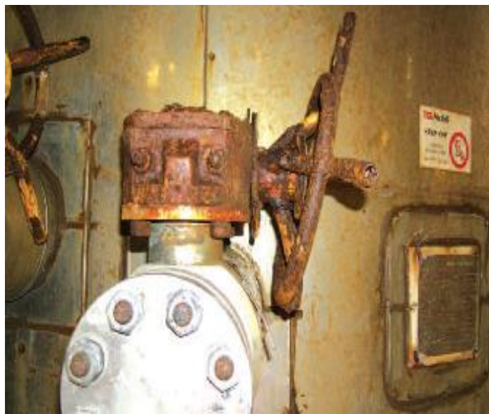
Figure 1-3. Corrosion of valve (Wintle and Sharp, 2008)
