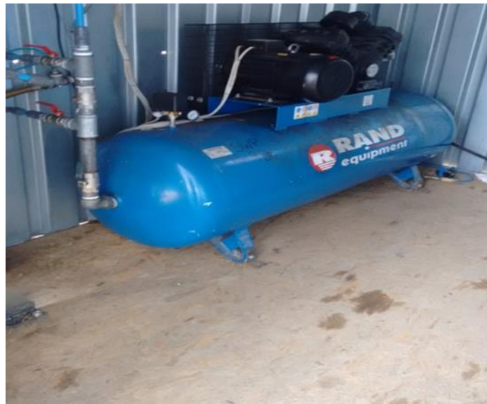
Figure 5-10 The air compressor for case study
