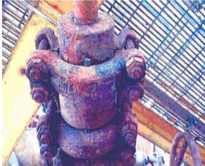
Figure 1-2 Corrosion of bolted connections (Wintle and Sharp, 2008)
