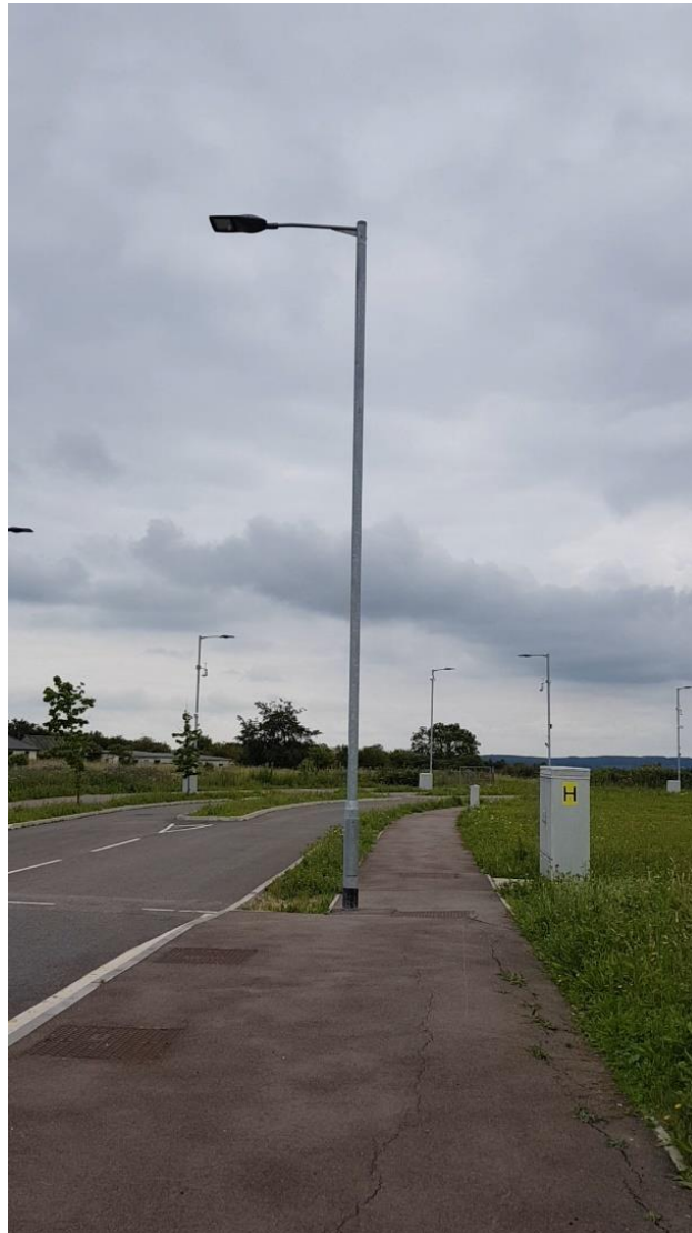
Figure 27 Light Pole studied
