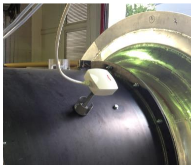
Figure 7-10 The Tempatron DP Series Installed in Segment 3
