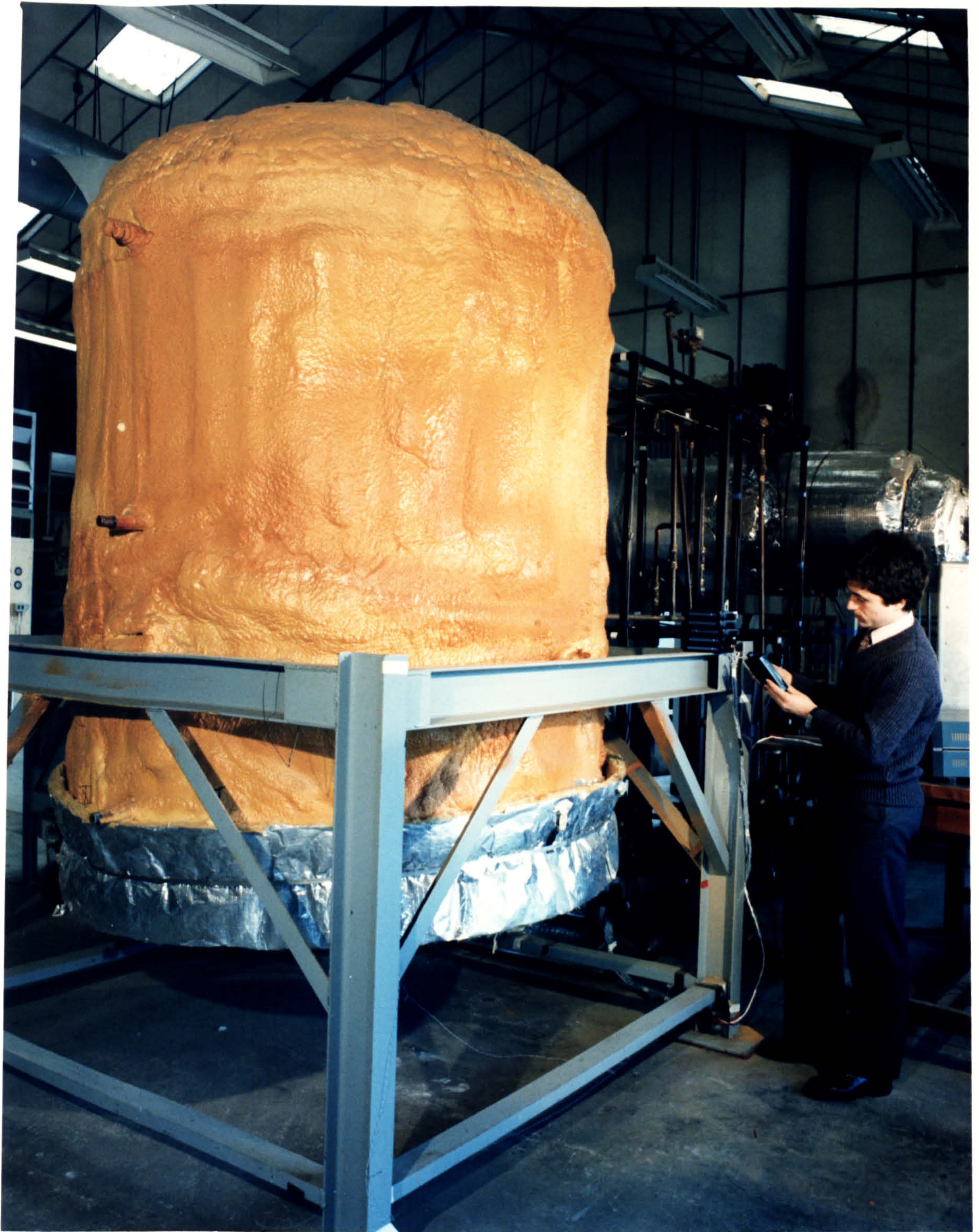
FIGURE 3.16 THE HOT WATER STORAGE VESSEL INSULATED WITH FOAM
