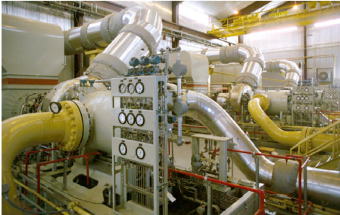
Figure 2-2 Typical Compressor Station [42]
