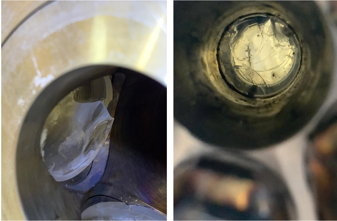
(a) inner view of glass. Layers of the material have broken off
