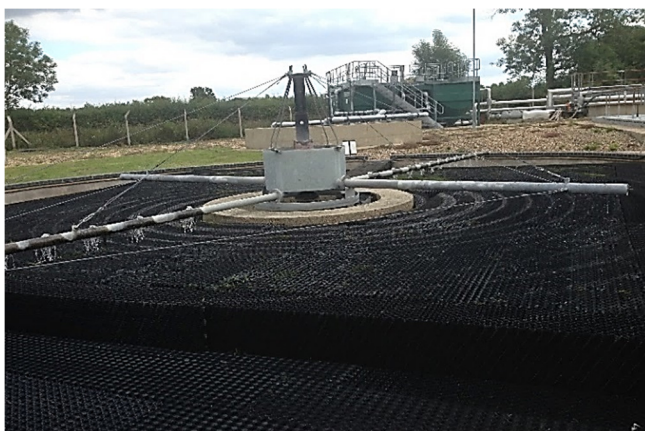
Figure 1: Cranfield wastewater treatment.
