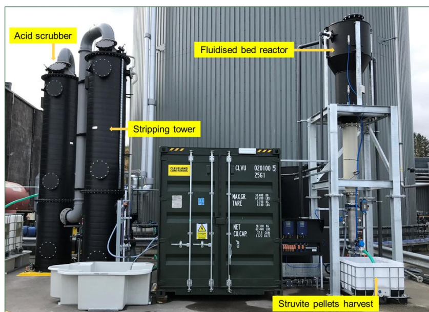
Figure 3-1. Above, flowsheet of the pilot scale treatment train treating digested distillery wastewater, comprising a fluidised bed reactor, ammonia stripping and scrubbing columns. Below, actual pilot scale treatment train, built and operated on site.
