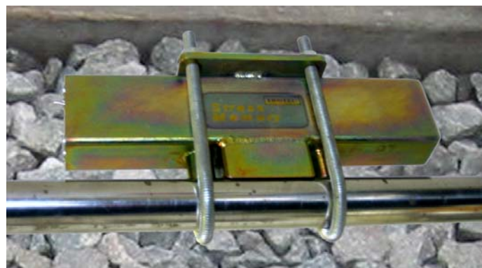
Figure 4: Railway Points Monitor
