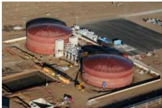
Fig.1. Andosol 3 Thermal storage tanks
