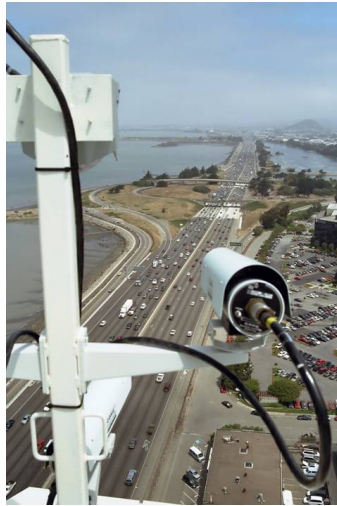
Figure 2-5 An illustration of the infrastructure-fixed camera in NGSIM [14].
